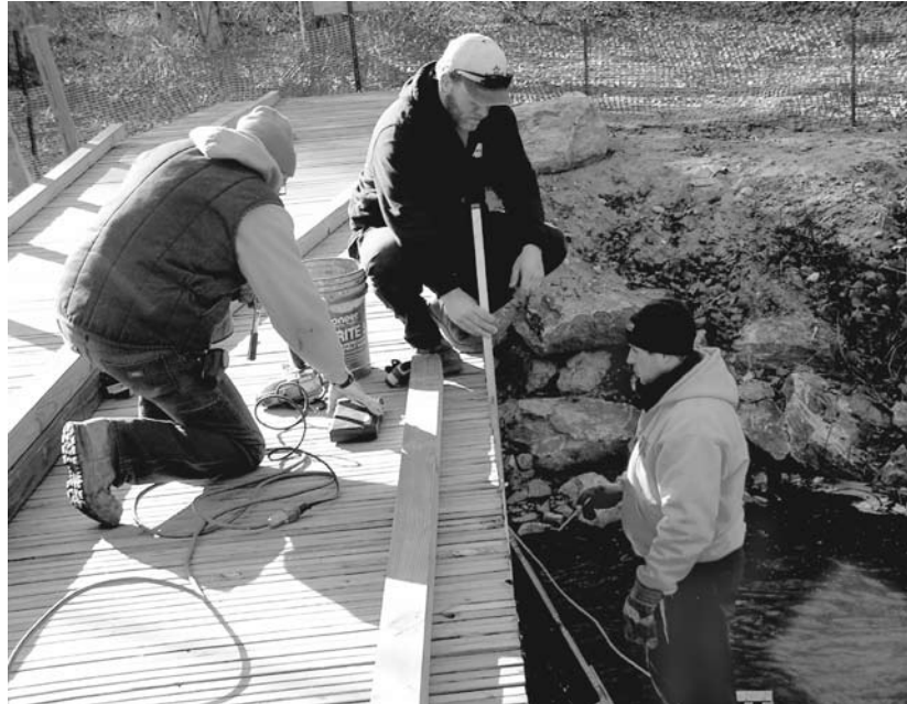
Town crews rebuilt the foot bridge at Salmon Brook Park using funds from a DEP grant to improve park use and access. We worked throughout the year and the finished product is both attractive and functional.
